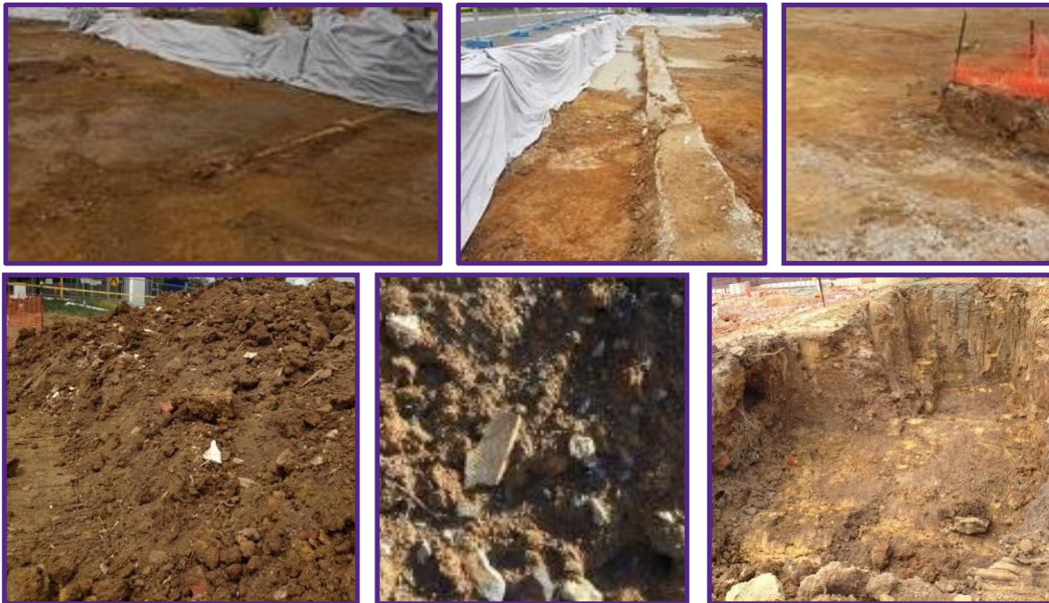
Figure 7.5: Pictures of the remediation program (top) and evidence of asbestos in soils (lower)
