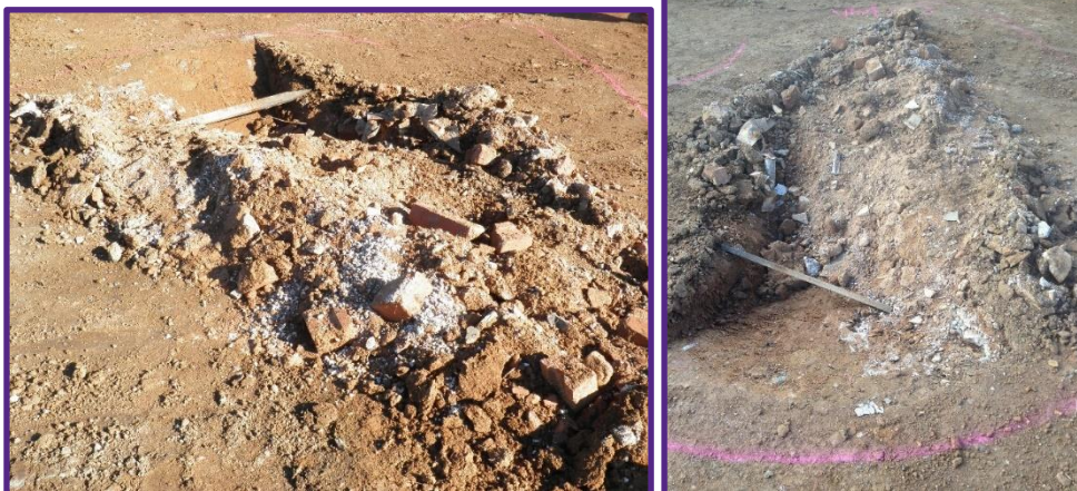
Figure 4.3: Asbestos contaminated soil found at the site
