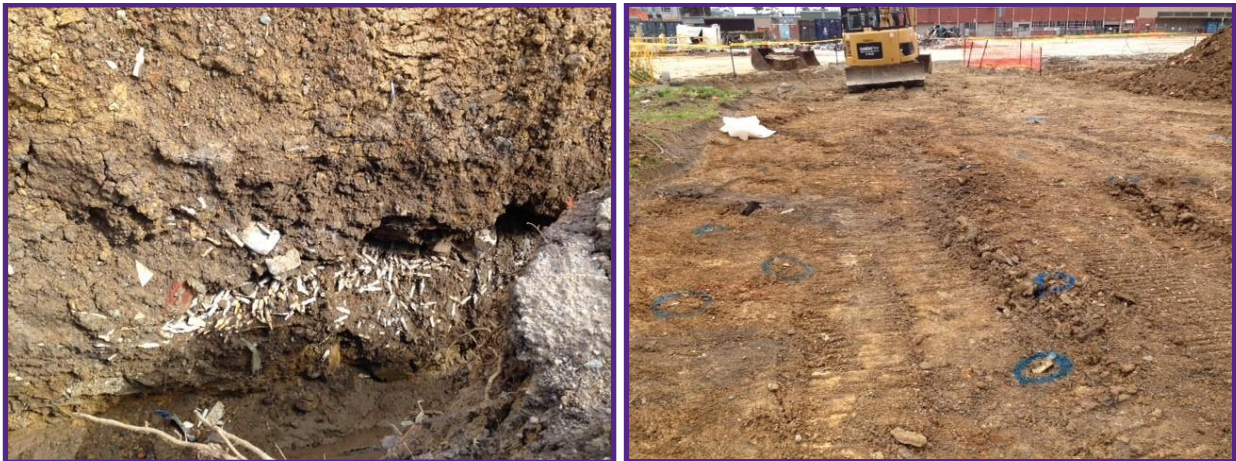
Figure 7.4: Asbestos contaminated soil found during the project (right image has asbestos circled in blue)
