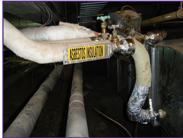
Figure 3.3 – Part of the remaining asbestos-lagged pipework
