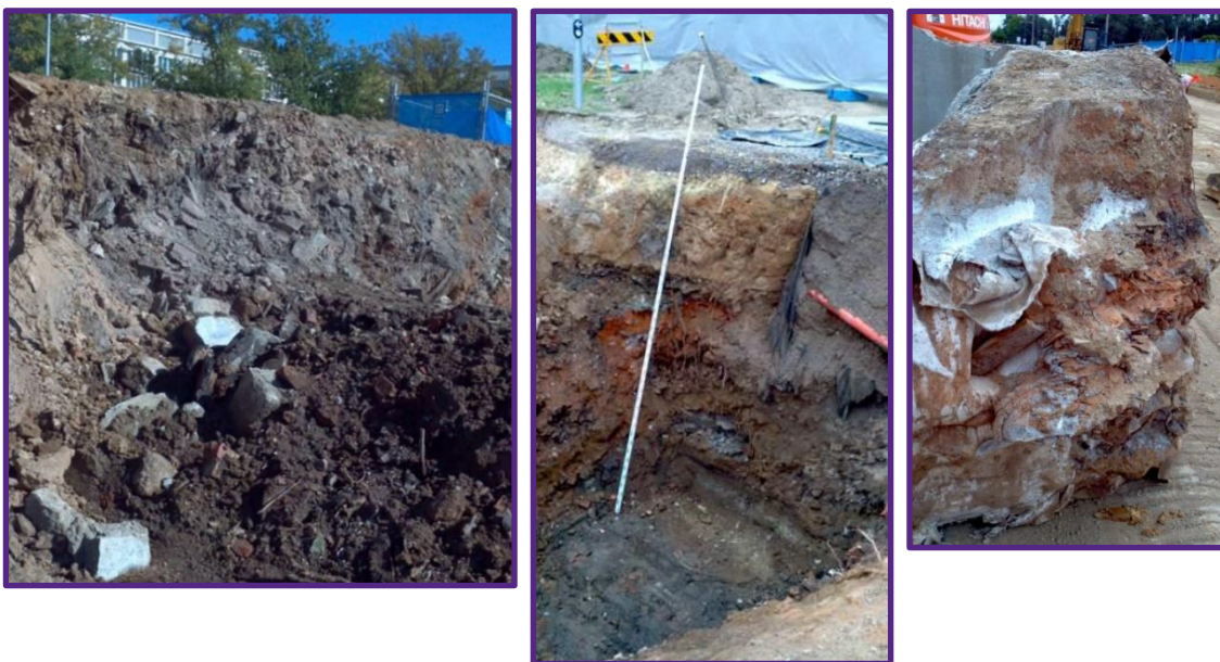
Figure 1.4: Asbestos contaminated soil along the southern boundary of the site (left image), an excavated section with up to 4 metres of highly contaminated soil underground (middle image, note the staff is 5 metres long), and asbestos containing material stuck to the outside of a concrete structure that was removed from the ground (right image)
