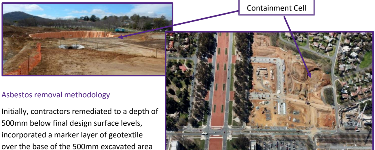
Figure 1.3: Construction of a 10,000 m 3 containment cell for low risk BRU material (left image), and the site in August 2014 (right image), with remediation complete on all subdivision blocks while infrastructure works were progressing.
