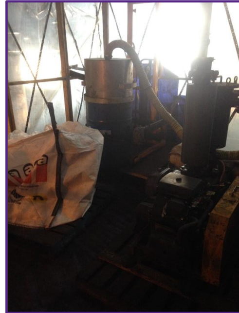
Figure 3.7 – Vacuum unit located inside the enclosure
