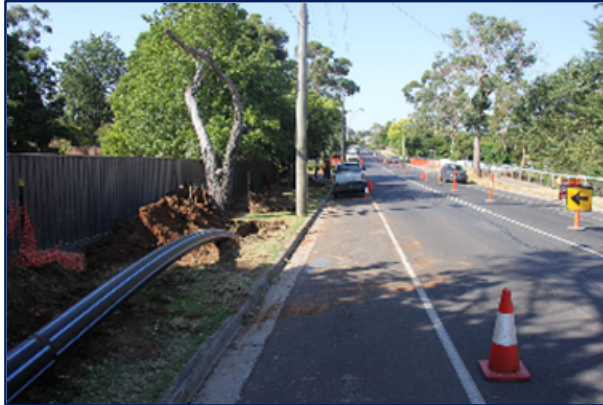
Photos: South East Water using the realign and leave method for pipe renewal.
