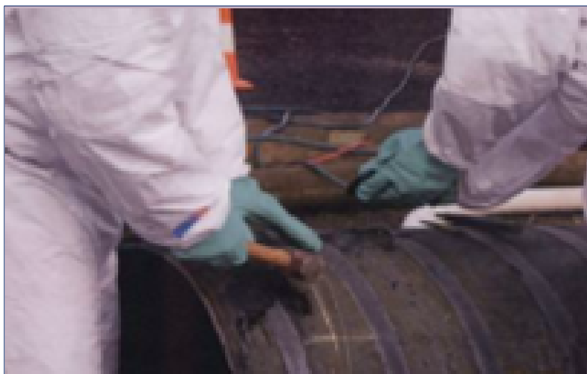
Photo: The hammer and chisel method used to remove asbestos from MSCL pipes.
