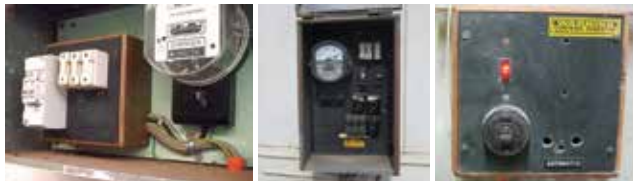
Figure 1: Asbestos based resin mounting boards used across Australia.
