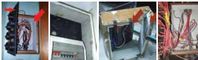
Figure 2: Asbestos cement and asbestos insulation mixed linings inside the electrical box itself.
