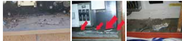
Figure 5: Asbestos millboard, asbestos resin board debris and asbestos insulation board debris in the bottom of electrical cabinets.
