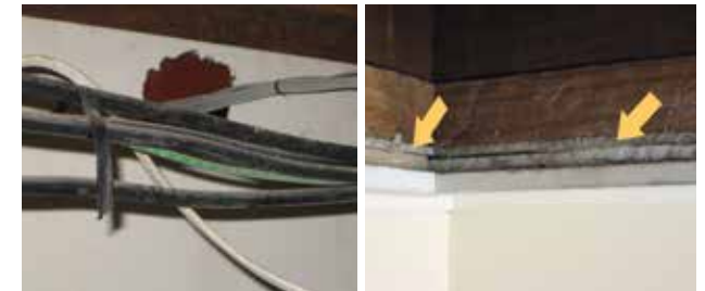
Figure 7: Take appropriate safety precautions including P.P.E. when running cables through asbestos and do not leave an asbestos mess for next time. The ongoing renovation boom in Australia has resulted in asbestos-containing materials being hidden to be found later by another tradesperson.
