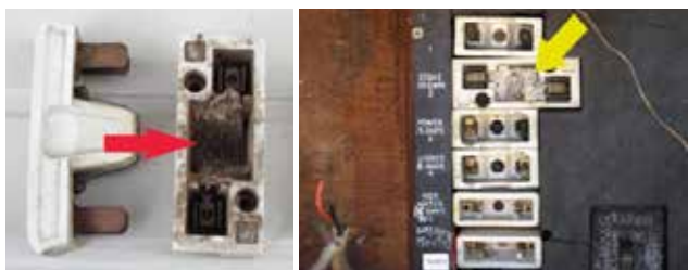
Figure 3: Woven asbestos textile fuse linings are common for large and small fuses.
