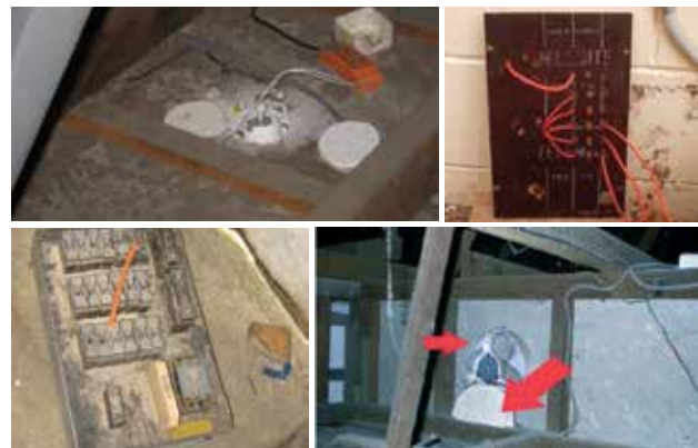
Figure 6: Discarded asbestos waste onsite. Often you will find asbestos debris discarded such as this asbestos insulation board ceiling pieces left lying in the roof, discarded electrical backing board, entire fuse box and asbestos cement pieces where a ceiling extractor has been installed.
