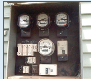
Electrical meter backing boards
