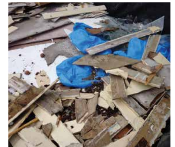
Figure 20: Multiple pieces of suspected ACM sheets in skip bin – evidence of poor removal methods being targeted as part of the audit program
