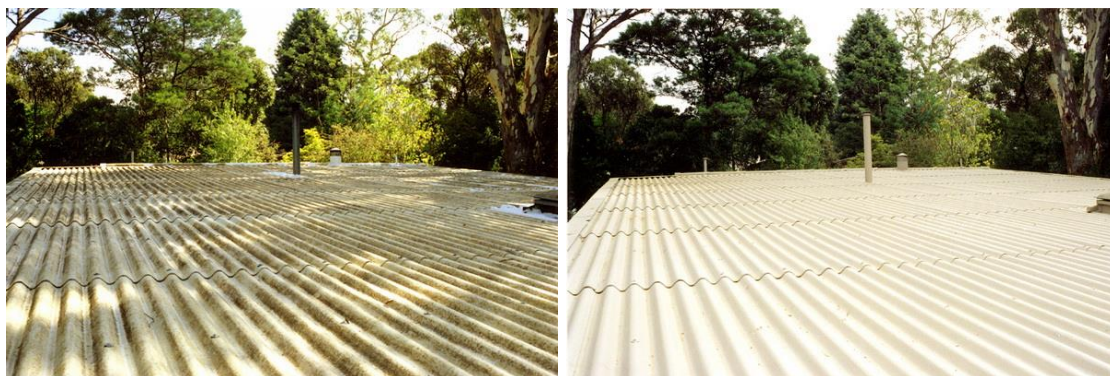
Figure 1: Photographs showing the application of an encapsulation product to an asbestos roof 17
