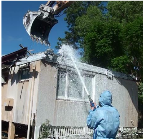
Figure 2: Use of Foamshield to encapsulate a fire damaged house prior to and during demolition 22
