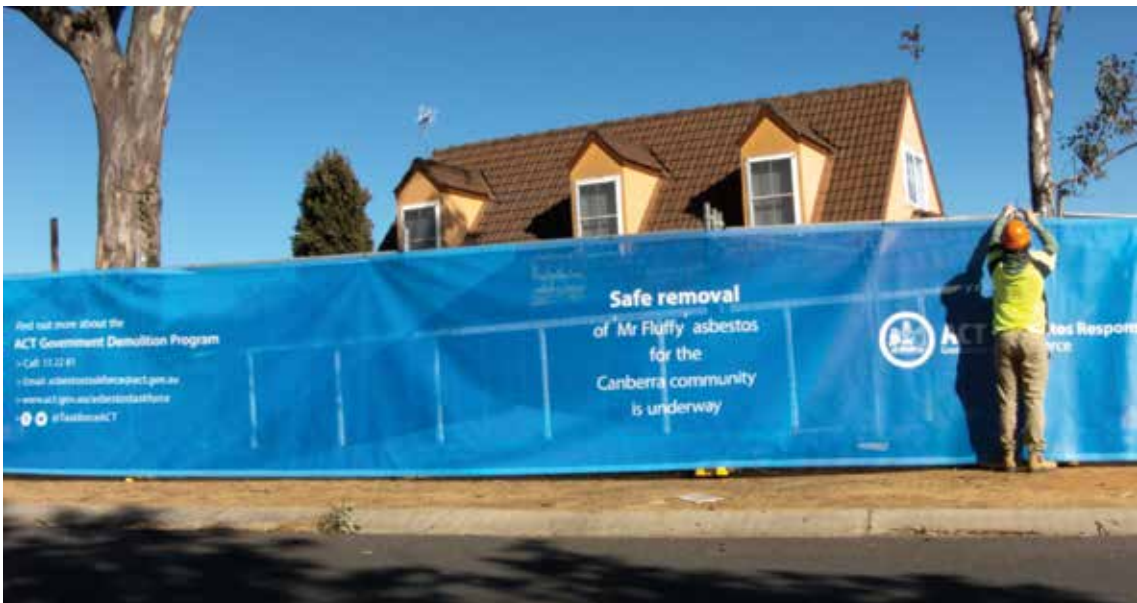
Images supplied from ACT Asbestos Response Taskforce
