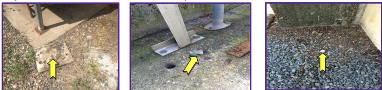
Figure 3.2: Asbestos debris from the storm was spread around the site
