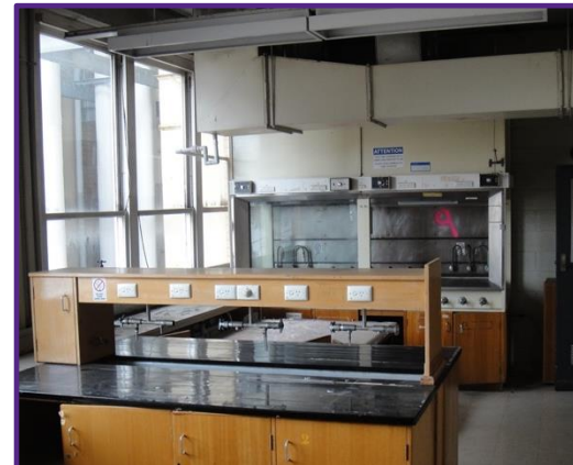
Figure 7.6: Risks were present in ventilation ducting, sinks and fumehoods
