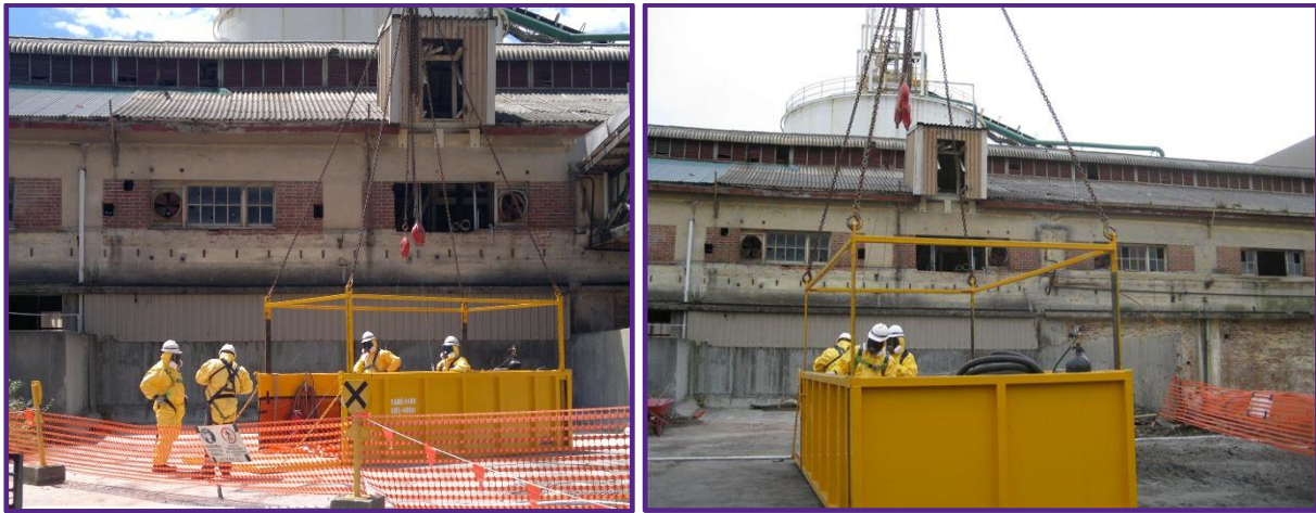
Figure 9.4: The crane and container used to hoist asbestos removal staff onto the roof for safe removal of asbestos
