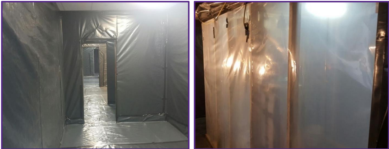
Figure 5.4: Plastic lining set up for asbestos removal (left picture) and the outside of a decontamination unit (right picture) 10
