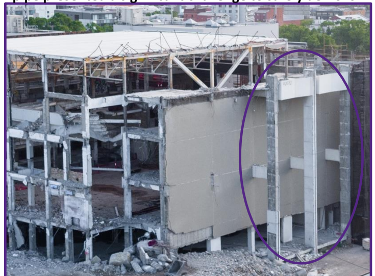
Figure 4.6: The 22-metre-high columns containing asbestos pipe presented a significant challenge to safely demolish
