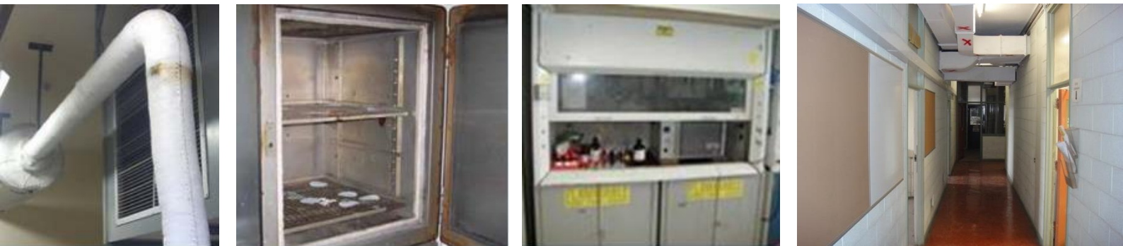
Figure 7.3: Asbestos was found in several areas including pipe insulation, kilns, fume cupboards and vinyl flooring
