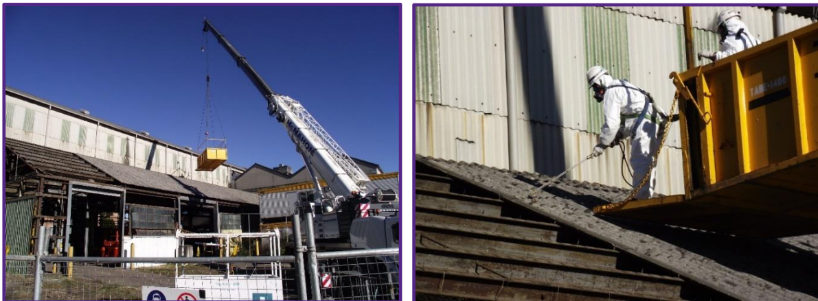
Figure 2.3: Purpose built aerial works platform and surrounding exclusion zone used to remove the asbestos roof and wall sheeting
