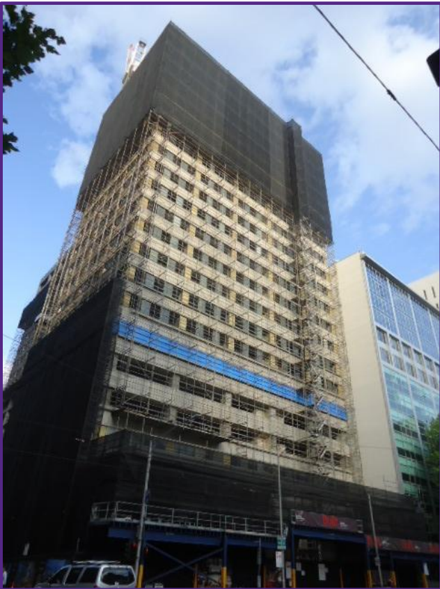
Figure 6.2: Asbestos containing materials were found in a number of areas, including the infill material between the exterior concrete panels
