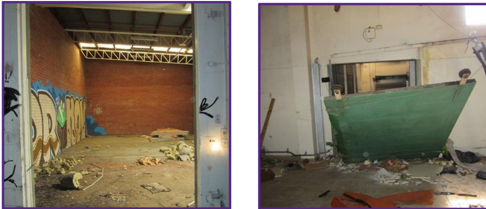
Figure 1.2: Abandoned site prior to clean up and asbestos removal
