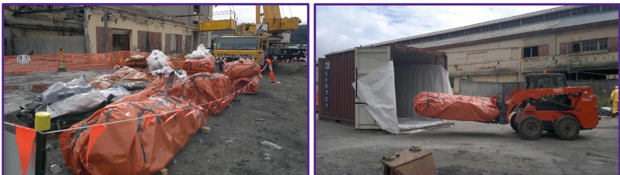
Figure 9.2: Asbestos contaminated items wrapped in plastic marked with asbestos signage (left image) prior to transportation to Brisbane via shipping containers (right image) for treatment and disposal
