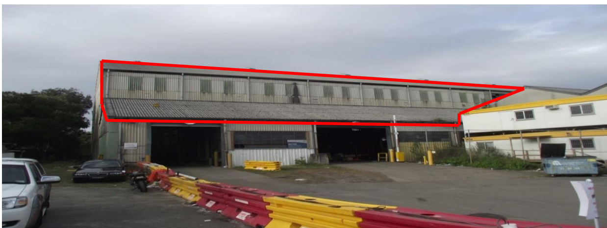
Figure 2.2: An example of asbestos roof and wall sheeting from the B5 Mill
