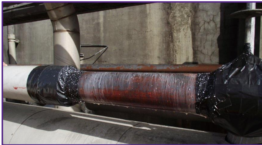
Figure 2.5: The finished clean section of the pipe insulation with a PVA solution
