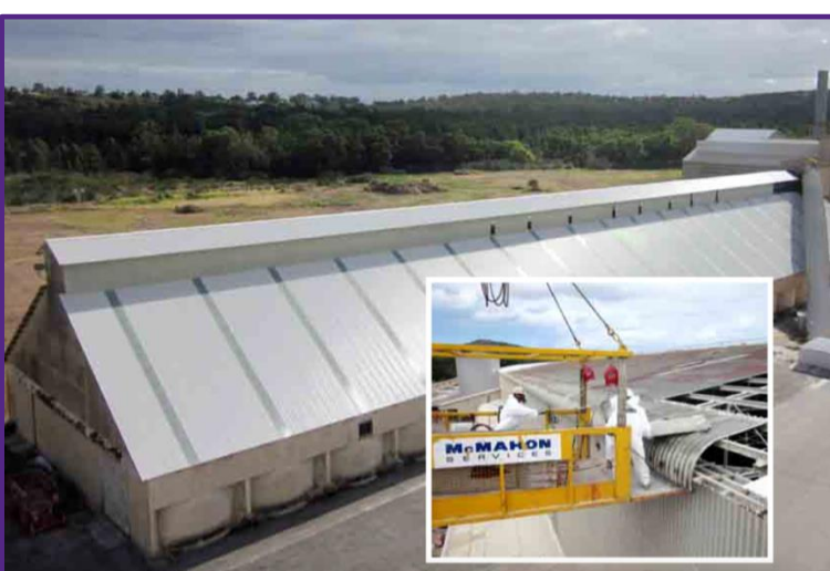
Figure 11.3: Removalists worked from the side of a cage utilising fall protection equipment
