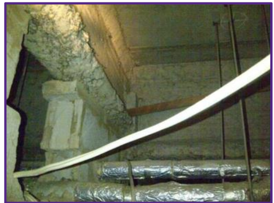
Figure 4.2: Significantly deteriorated asbestos insulation found directly above cinderblock wall which was built directly up to the base of the insulation
